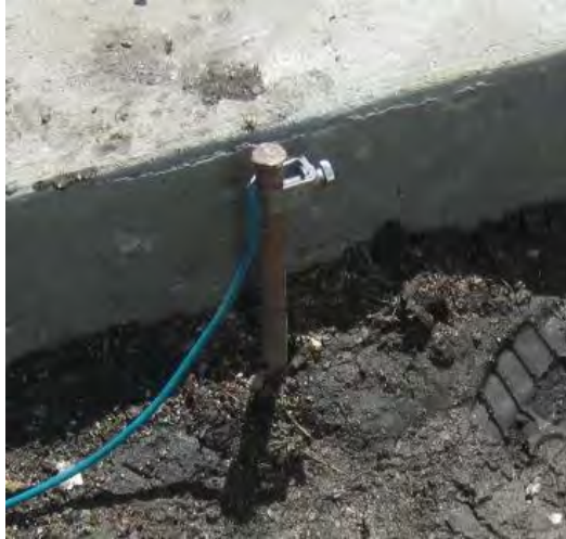
Image 2-5 – Ground rod, buried
