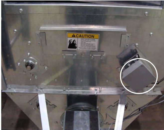
Image 4-20 – Meter roll proximity switch box
