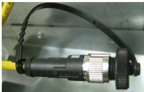
Image 4-39 – Moisture sensor cord capped
