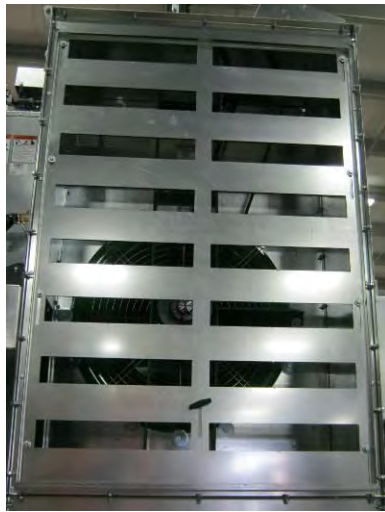
Image 37 – Air inlet louvers
