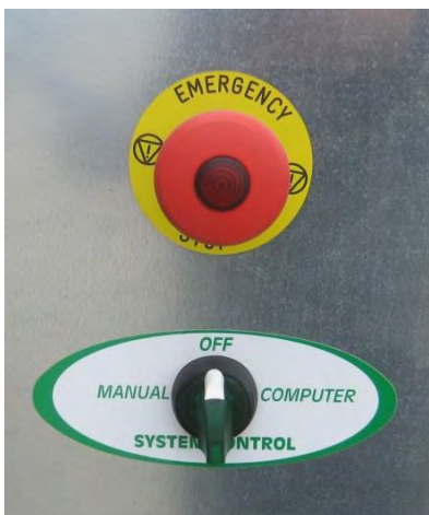
Image 3 – Emergency stop and system control switch
