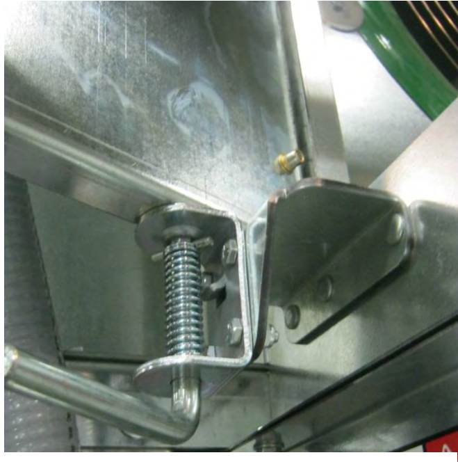
Image 3-4 – Spring pin on intake door
