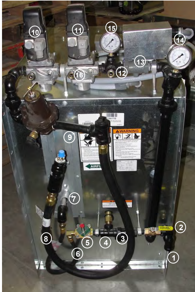
Image 7 – Pipe train components
