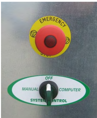
Image 22 – Emergency stop button and system control switch
