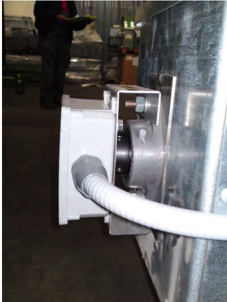
Image 4-4 – Unload auger proximity switch
