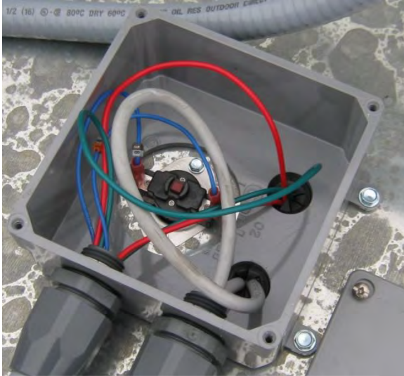
Image 4-9 – Heater housing hi-limit switch
