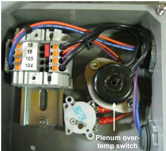
Image 4-14 – Plenum over-temperature switch
