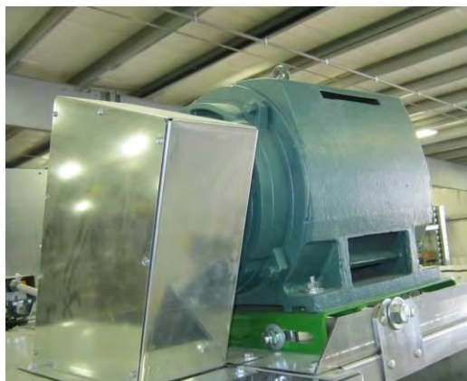
Image 38 – Fan motor and drive shield
